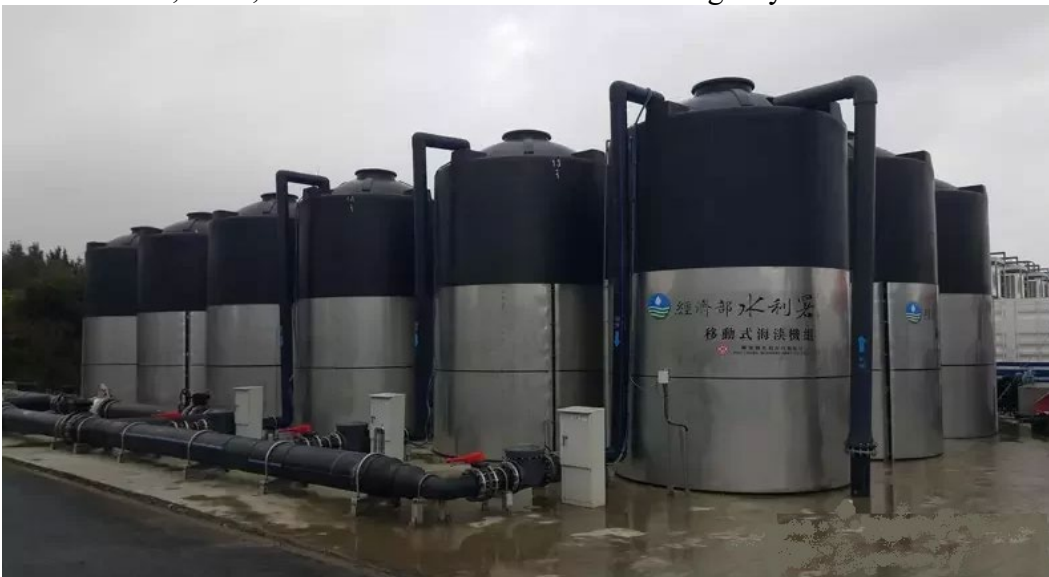
Water production and delivery facilities
