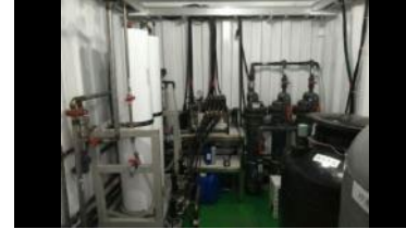
Inside of Container 貨櫃內設備
